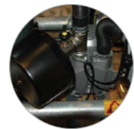
Inlet blower filters
