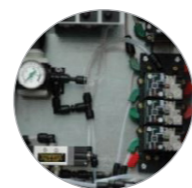
Pneumatic control systems
